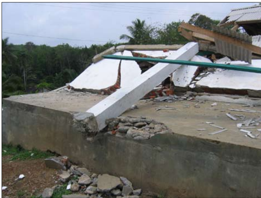
Figure 20. Collapsed confined masonry building, note lack of plinth beam and connection between column and plinth, Pal 30, Kec. Lais, (North Bengkulu), S3.53490° E102.05996°.
