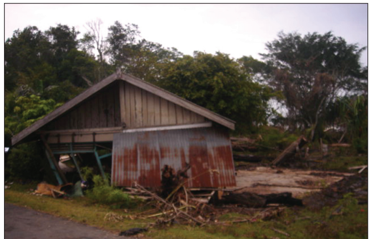
Figure 2. House pushed off its foundation by the tsunami at the coast of Serangai Village in Batik Nau District, south part of Mukomuko Regency, S3.2538^\circ E101.5335^\circ (photo: Karnawati).
