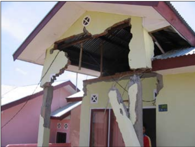
Figure 8. Subdivision of confined masonry houses, damage to covered terrace, Bengkulu, S3.83218° E102.29287°.
