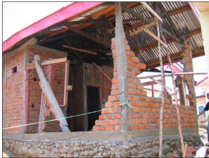
Figure 9. Subdivision of confined masonry houses, collapse of masonry wall exacerbated by insufficient connections, Bengkulu, S3.83218° E102.29287°.
