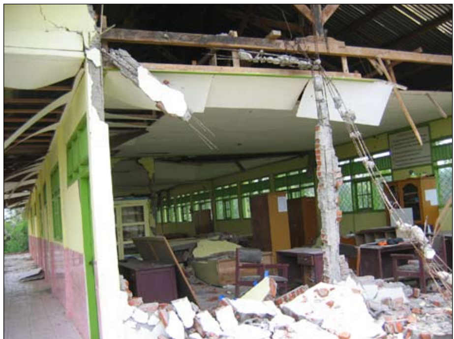
Figure 19. Sekolah Dasar Negeri No. 04, note steel splice location, use of rounded cobbles in concrete, Kec. Lais (Bengkulu), S3.52958° E102.04525°.
