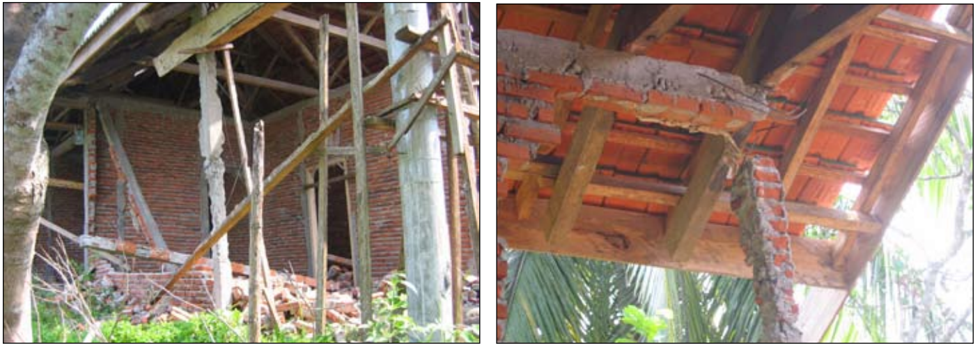
Figure 3. Confined masonry houses with failure in masonry walls and connections between tie columns and bond beams, Kec. Airnapal (North Bengkulu).
