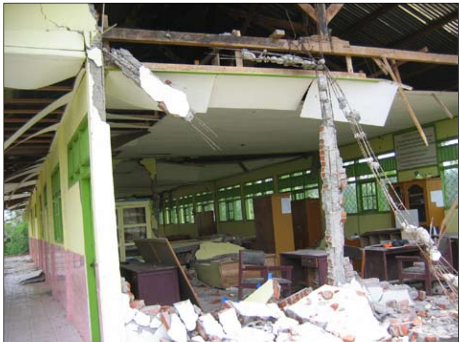
Figure 19. Sekolah Dasar Negeri No. 04, note steel splice location, use of rounded cobbles in concrete, Kec. Lais (Bengkulu), S3.52958° E102.04525°.
