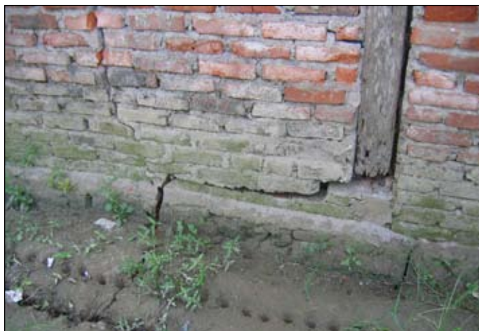
Figure 13. Cracks in foundation and walls associated with settlement and tilt on liquefiable soils, Lempuing (Bengkulu), S3.82799° E102.28473°
