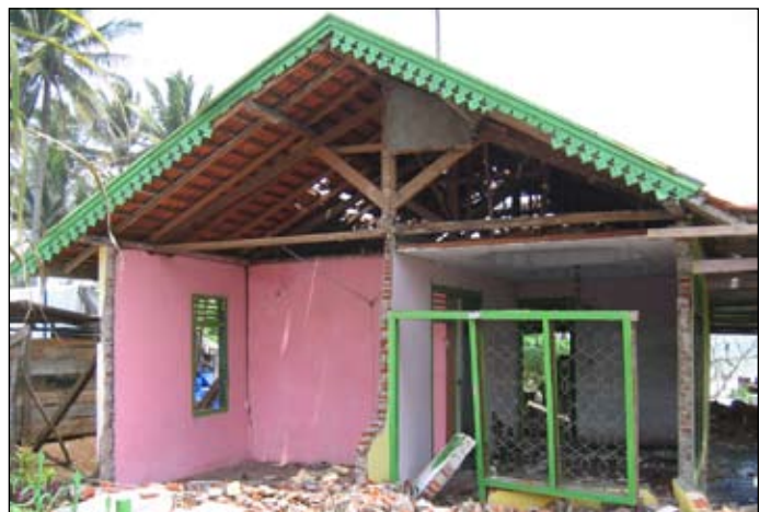
Figure 5. Partially collapsed brick masonry house with RC tie columns and timber bond beams. Note partial collapse of masonry gable wall and lack of inplane stiffness in front wall, Kec. Lais (North Bengkulu), S3.53217° E102.03771°.
