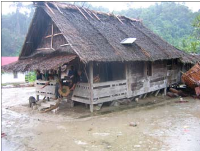
Figure 11. Timber frame with posts resting directly on soft ground, Barimanua, Pulau Sipora, Mentawai Islands.
