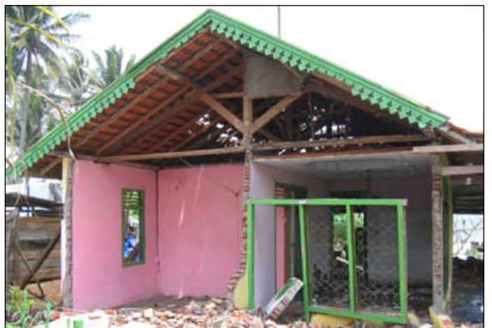
Figure 5. Partially collapsed brick masonry house with RC tie columns and timber bond beams. Note partial collapse of masonry gable wall and lack of inplane stiffness in front wall, Kec. Lais (North Bengkulu), S3.53217° E102.03771°.
