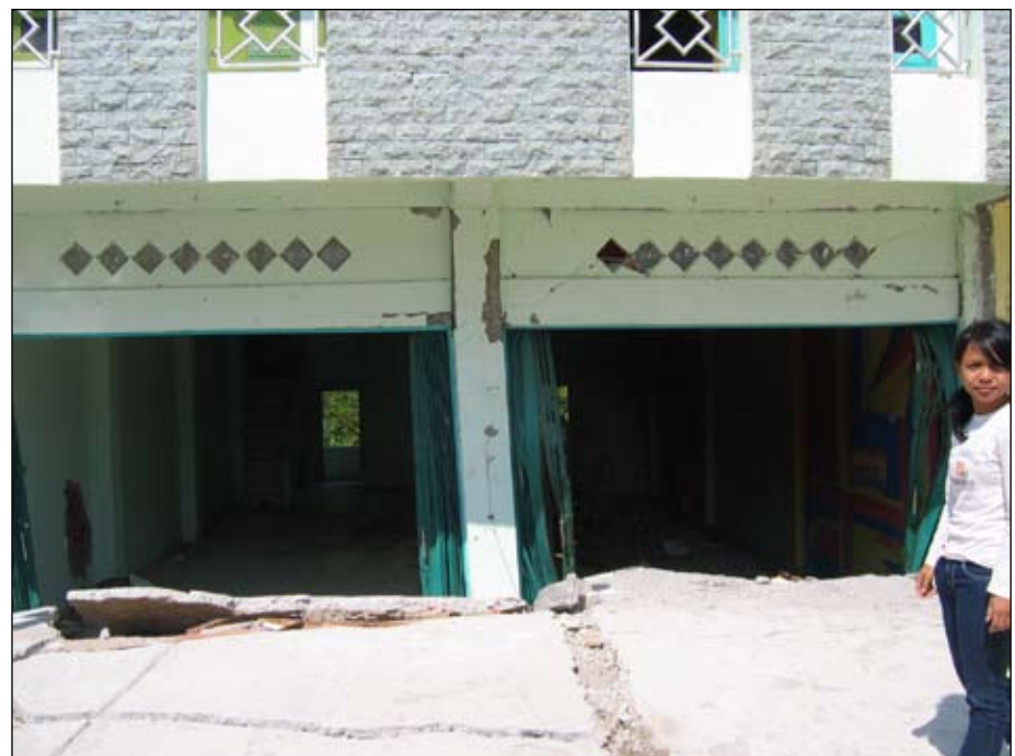
Figure 16. Two-story ruko, 3° tilt in first floor column, Bengkulu, S3.80362° E102.27617°.
