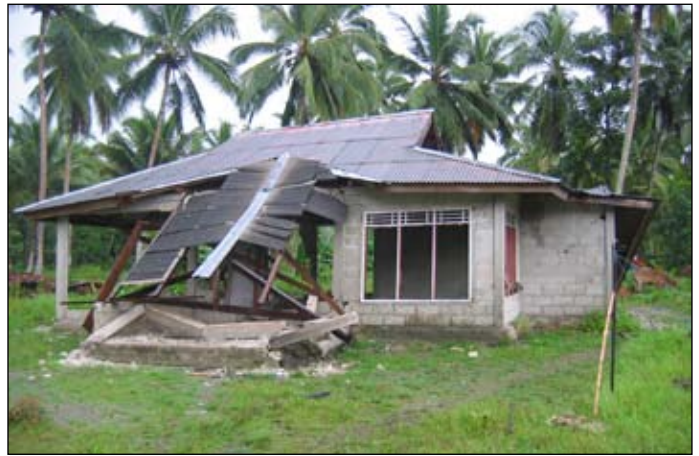
Figure 12. Confined concrete block masonry, partial collapse due to lack of sufficient connections between confining elements, Barimanua, Pulau Sipora, Mentawai Islands.
