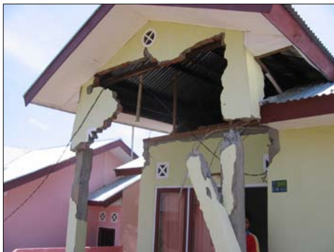
Figure 8. Subdivision of confined masonry houses, damage to covered terrace, Bengkulu, S3.83218° E102.29287°.
