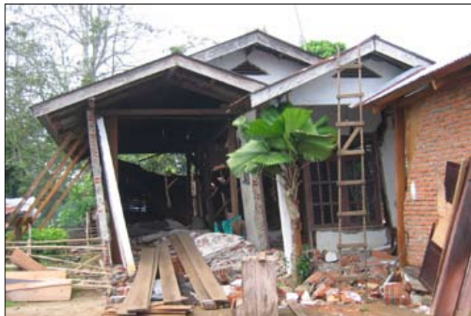
Figure 4. Partially collapsed unreinforced masonry house with timber bond beam (North Bengkulu).
