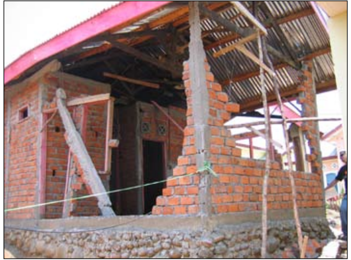
Figure 9. Subdivision of confined masonry houses, collapse of masonry wall exacerbated by insufficient connections, Bengkulu, S3.83218° E102.29287°.
