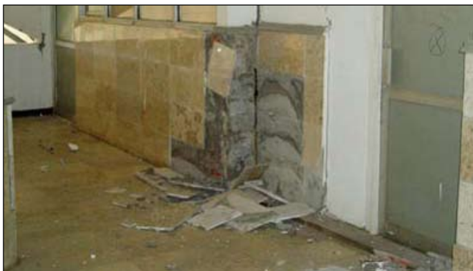
Figure 21. Nonstructural damage at M. Yunus hospital in Bengkulu (photo: Boen).
