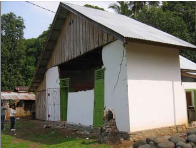
Figure 6. Confined masonry house with failure in masonry walls and connections between tie columns and bond beams, Kec. Airnapal (North Bengkulu).
