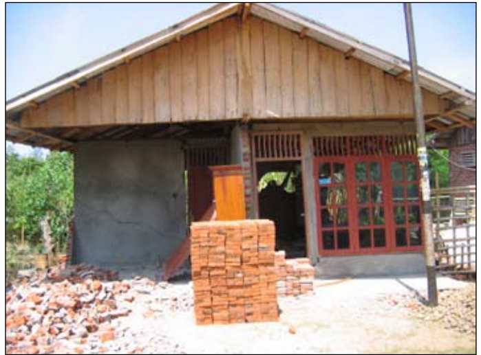
Figure 7. Partially collapsed unreinforced masonry house with timber bond beam, Lempuing (Bengkulu), S3.82799° E102.28473°.
