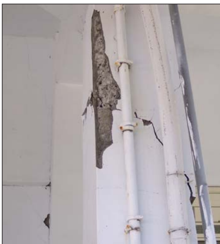
Figure 10. Shear cracks due to the short column effect.
