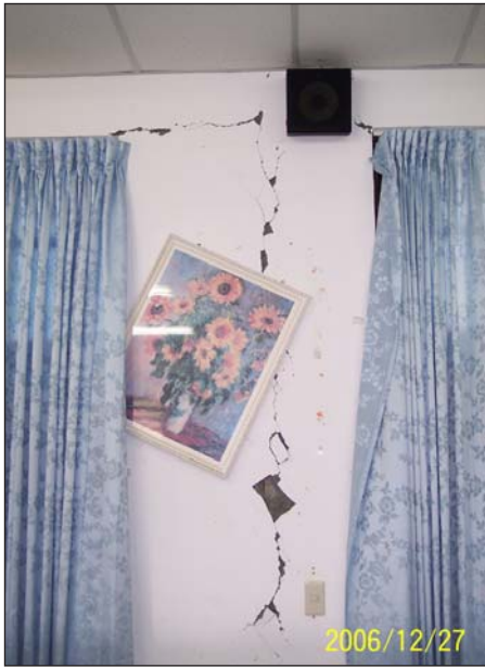
Figure 9. The damaged column along the corridor.
