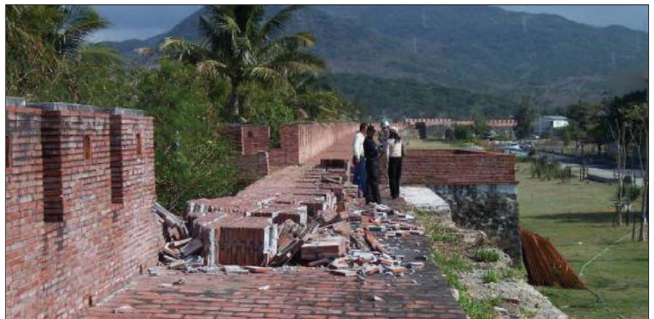
Figure 11. Collapsed battlements of the old city wall.
