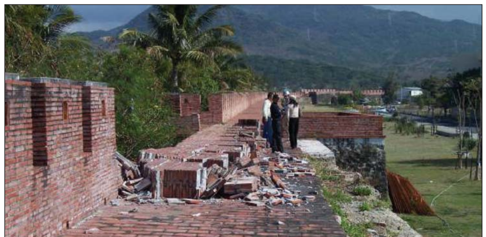
Figure 11. Collapsed battlements of the old city wall.
