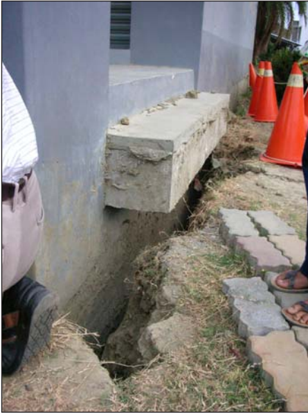
Figure 6. Ground settlements and lateral displacement observed in the Hengchun Elementary School.
