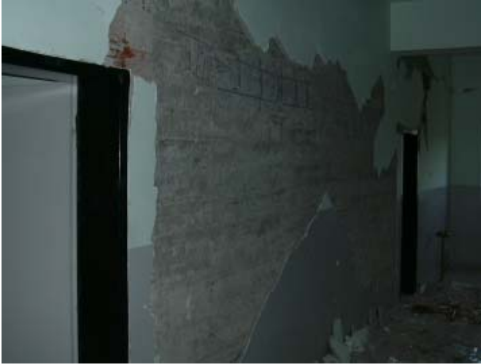
Figure 22. Just-Completed High School Building in City (The two shear walls flanking the hallway are the only ones in the longitudinal direction. Wall facing this one damaged worse. The only wall in the transverse direction appeared to be in a state similar to this. Source: Dr. E. Karaesmen.)
