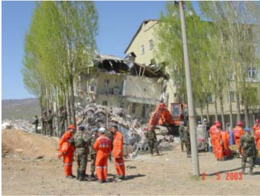
Figure 24. Collapsed Building at East Exit from City
