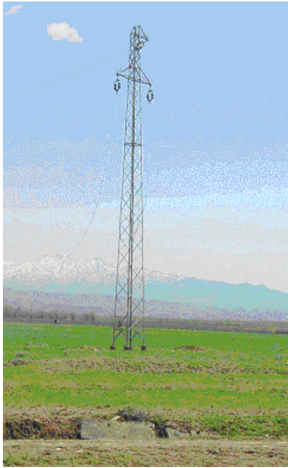
Figure 18. Power Pylon about 100 m Away from Çeltiksuyu School (Note loose alluvial soil and ground water seeping from ditch in foreground. This pylon had snapped the power cables on the west side. Soil here and at the school appeared to be S_E/S_F in the UBC characterization.)
