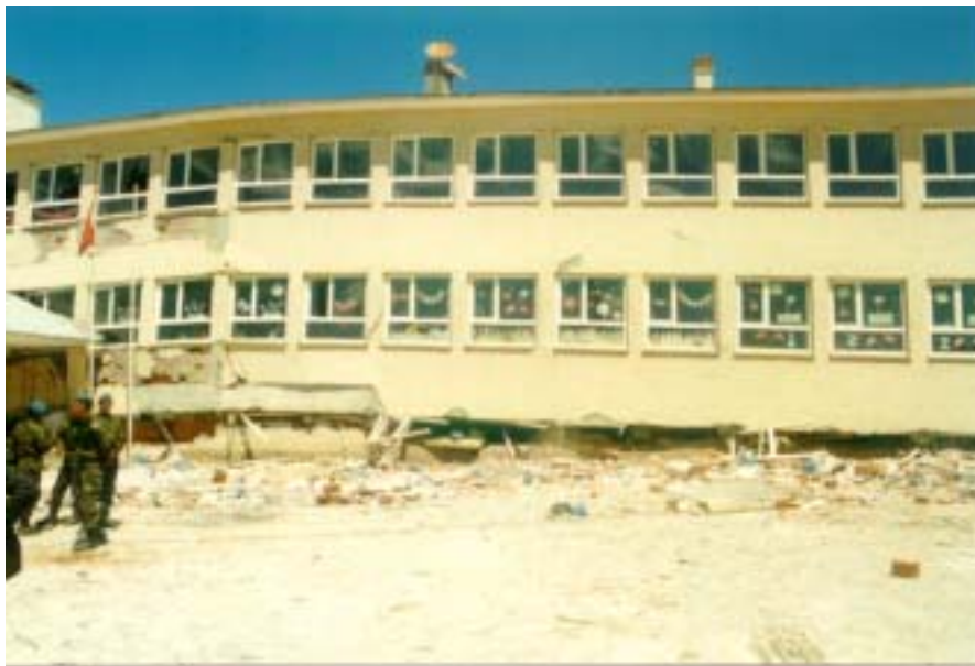
Figure 15. Çeltiksuyu Regional Primary Education School Building (Note identical entrance canopy partially visible on left. Again, the ground story had collapsed fully in exactly the same way as that in Figure 14. This building had been completed in 1998.)
