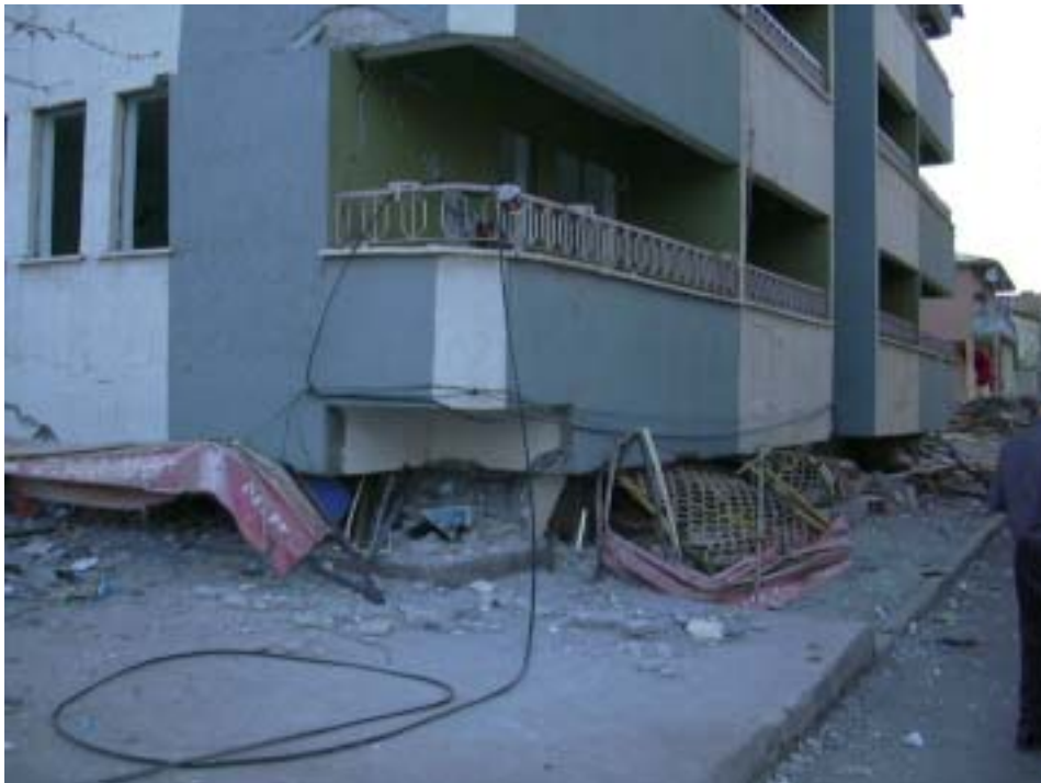
Figure 23. Another Recently Completed Building That Experienced Ground Story Failure (Source: Dr.E. Karaesmen)
