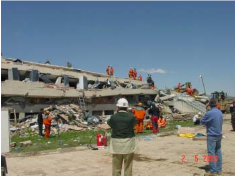
Figure 16. Dormitory Block on the west of the class room block at Çeltiksuyu Regional Primary Education School (All three stories appeared to have turned into mechanisms, resulting in complete pancake type collapse. Plain reinforcement was visible in broken columns.)
