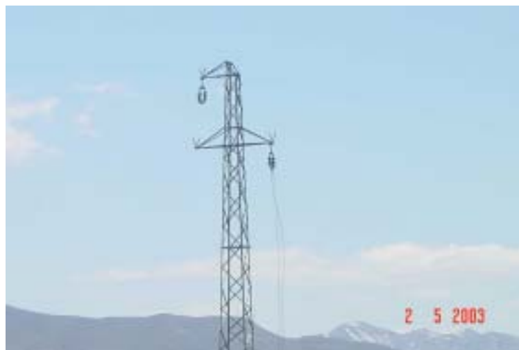
Figure 19. Pylon Immediately on West of That in Figure 18. (Could this have been an indication of an extremely powerful fling that caused the cables to rupture? The truss members appeared to be unaffected.)
