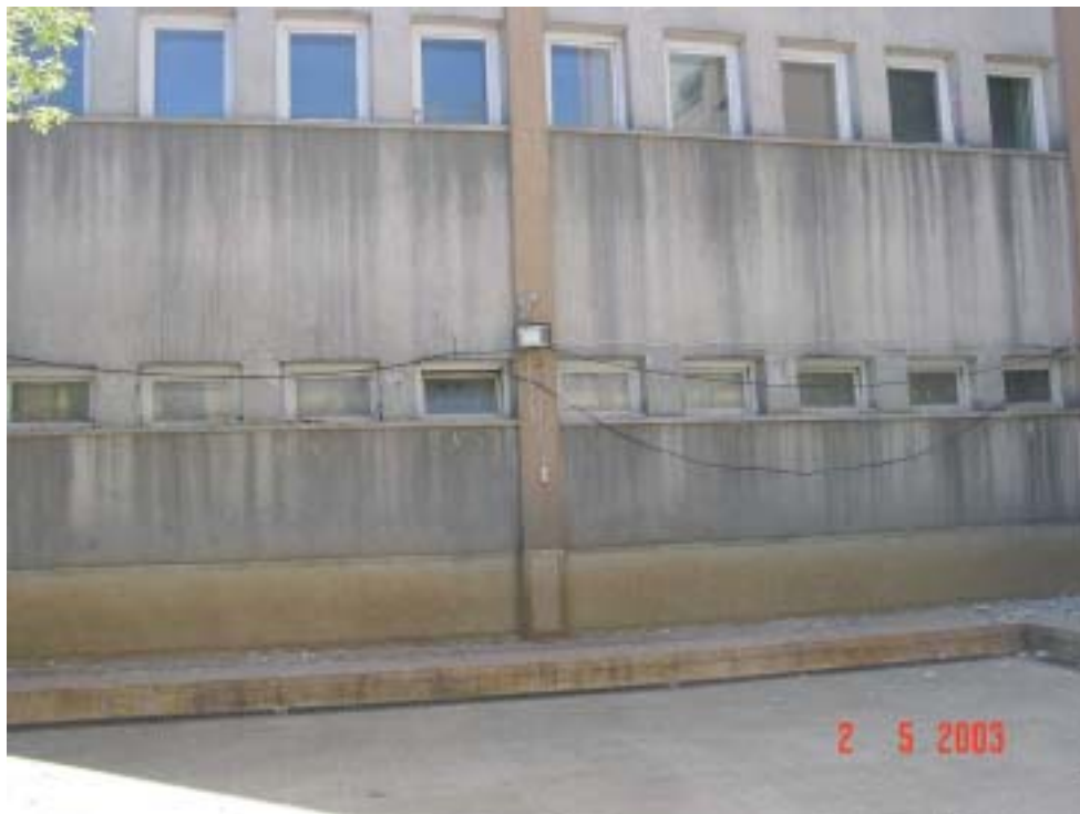
Figure 25. Regional Office Building of Public Works and Settlement from Inner Court (An identical replica in Bolu had suffered heavier damage in 1999 with column in middle shearing due to short column action. The situation here was one of impending failure in same way.)
