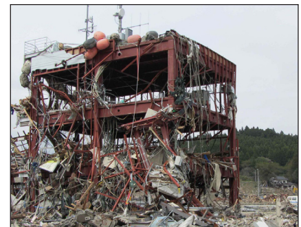
Damage from 2011 Tohoku, Japan, tsunami (photo: L. Dengler).
