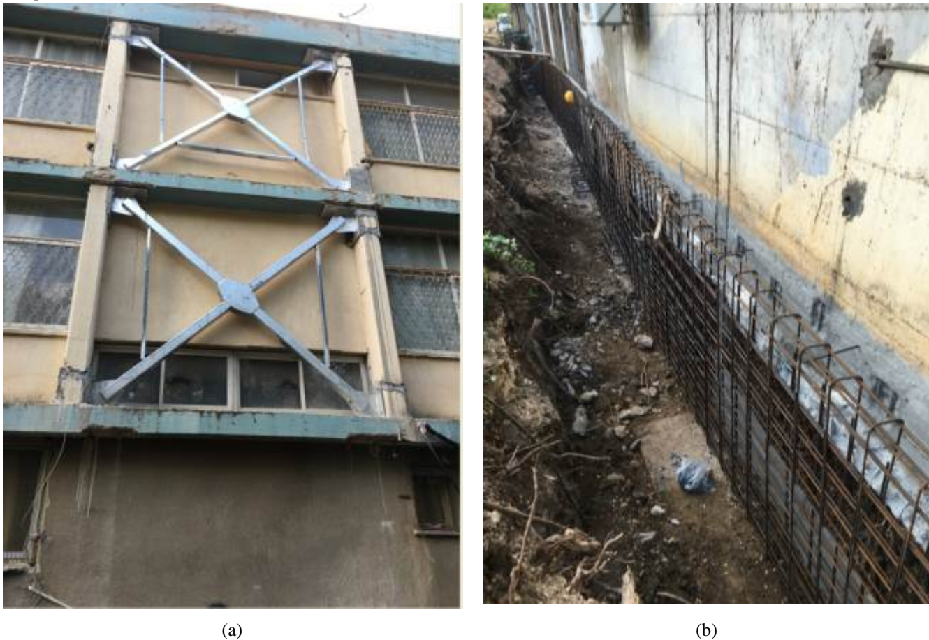
Fig. 5 – retrofit of Meginim School (Kiryat Shomna): (a) addition of yielding steel braces; (b) addition of grade-beam between foundation to reduce effects of potential ground rapture at surface level
